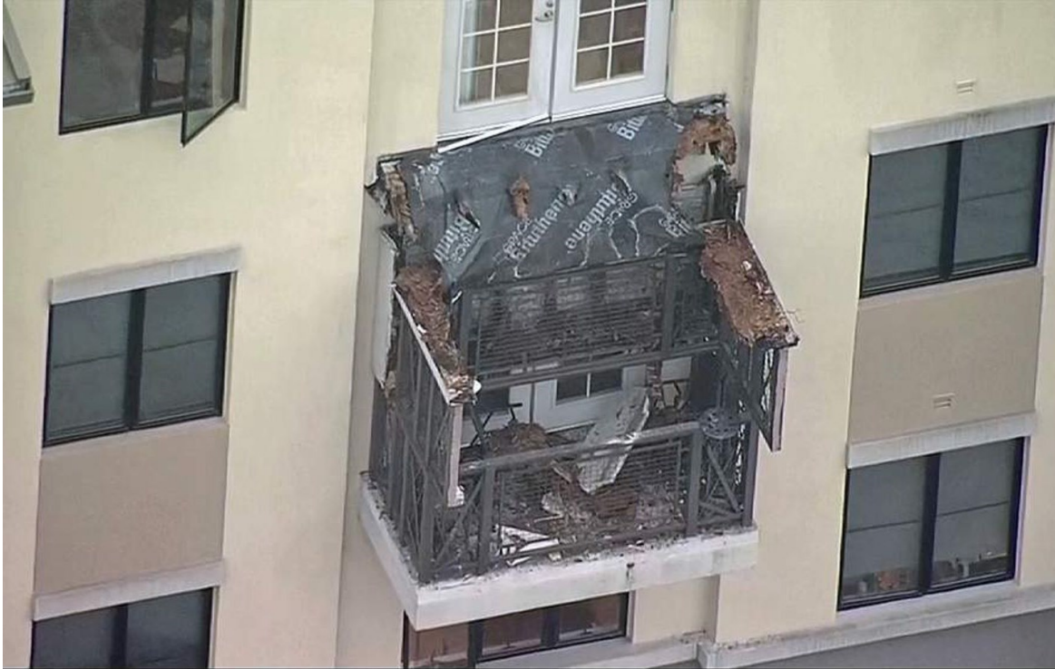
Balcony collapse in Berkeley, CA, leads to 6 fatalities
