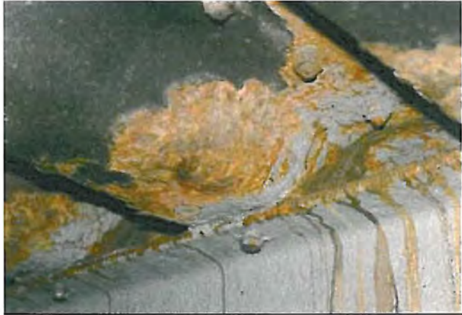
SEVERITY CODE 2 (1.1 and 1.3)
