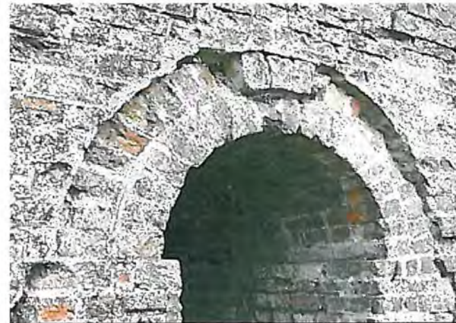
SEVERITY CODE 4 (3.3 and 3.6)
