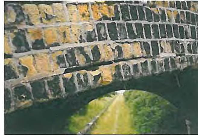
SEVERITY CODE 3 (3.2 and 3.3)
