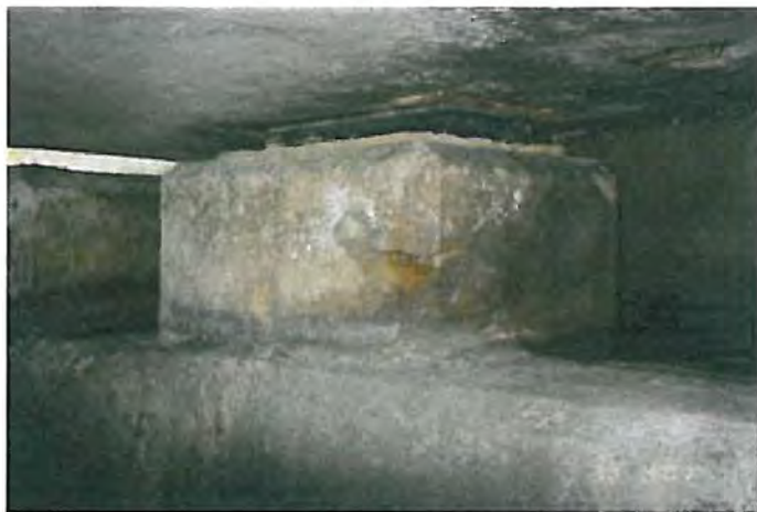
SEVERITY CODE 2 (bearing plinth/shelf - 2.2)
