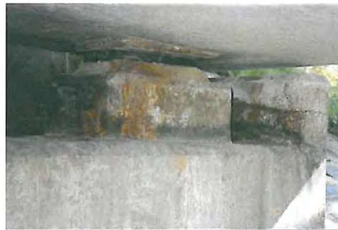
SEVERITY CODE 3 (bearing plinth/shelf - 2.2)
