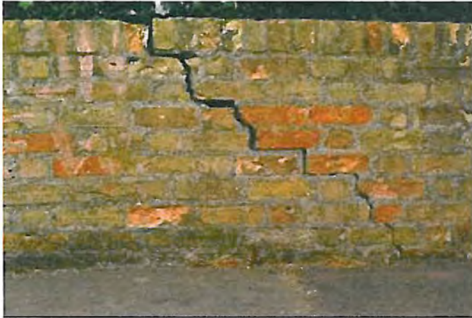
SEVERITY CODE 4 (3.5 and 3.7)
