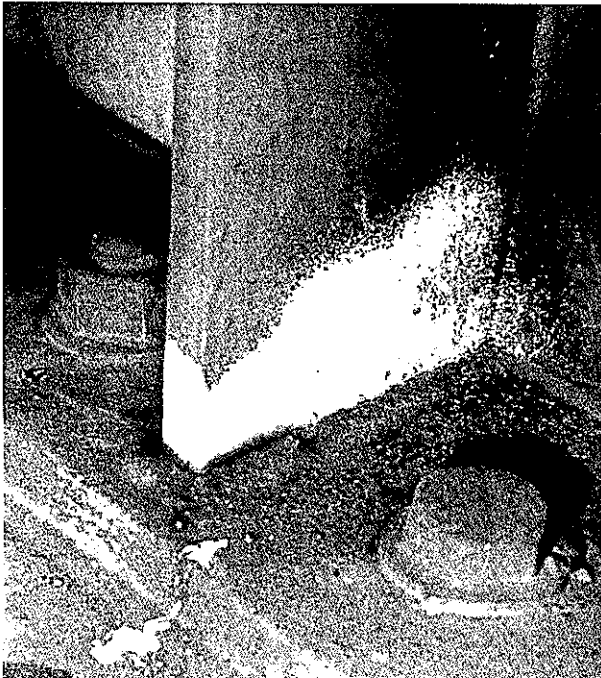
Plate 12. Crack at welded joint
